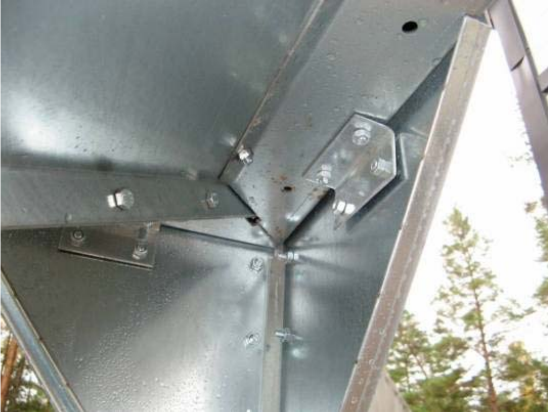
A photo showing the fastening of the central leg to the cone. The arrows point to the topmost row of perforation without bolts inserted.
