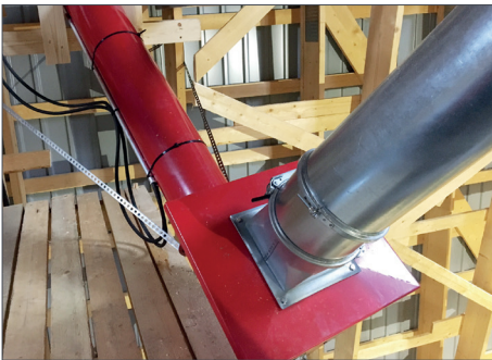
Hopper / 160mm/200mm pipe connection to the hopper
